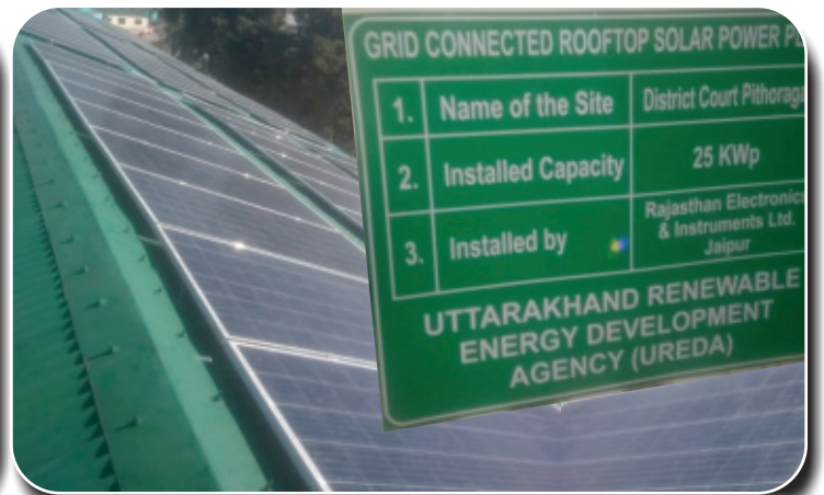
Cumulative 41 kWp Grid Connected SPV Power Plant at District Court Campus, Pithoragarh and Champawat
