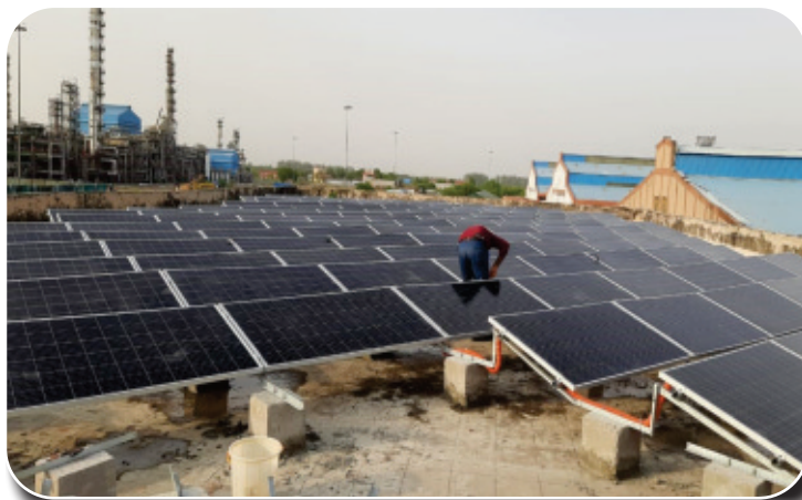
SPV Power Plant at GAIL PATA, Auraiya (UP)
